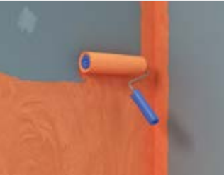
Figure 37: 2× full-surface application of fermacell Waterproofing Application with a roller (minimum total thickness 0.5 mm)
